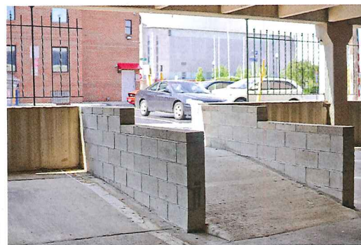
BELOW: The entrance ramp to West Lane Garage was retrofitted to accommodate motorcycle parking.
